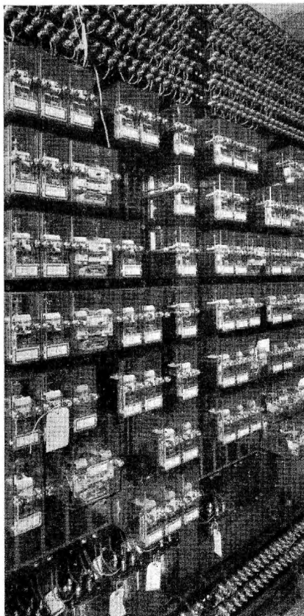
Below—Type B quick-detachable relays on board in tower Right—Rear of the board showing the wires and cables
