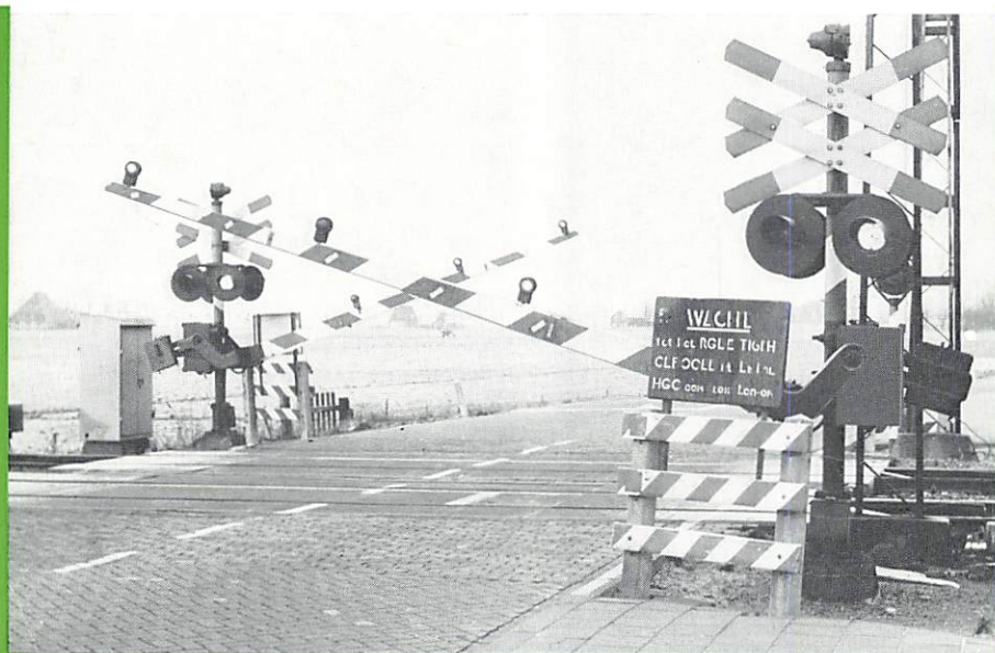
Automatic half-arm barrier installation with flashing lights on a double track.
