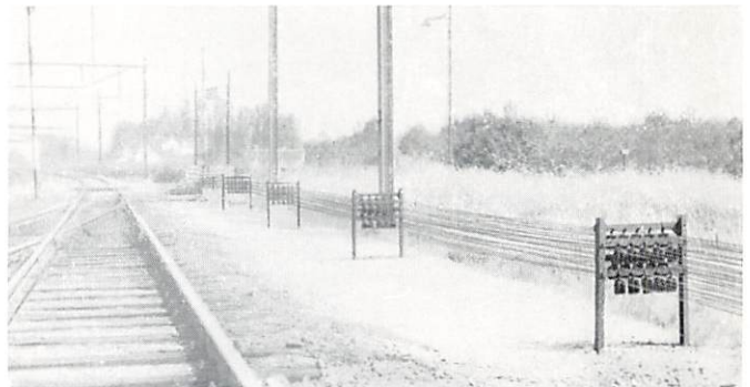
Above-ground wire arrangement.
